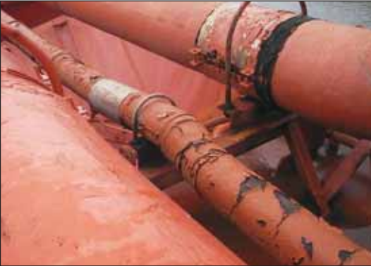
Areas of defect insulation, ready for upgrading
